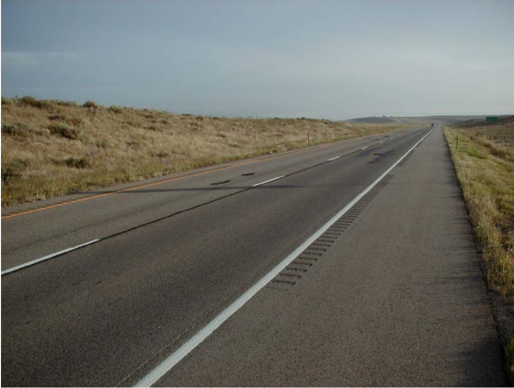
Figure 10. Typical EB Condition (9/24/05)
