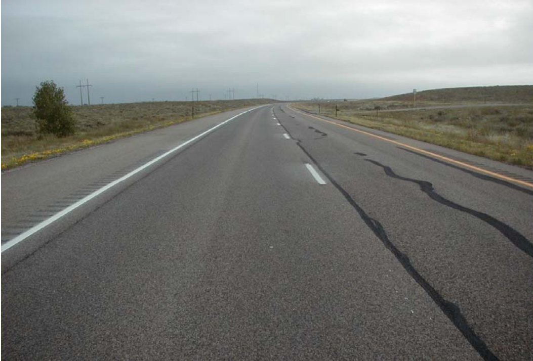
Figure 11. Typical WB Condition (9/24/05)
