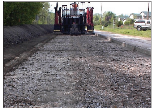
Existing concrete pavement on a rural highway in Kenosha County is rubblized in place and used as a base course. The county saved about 40 percent in estimated costs on a recent highway project.
