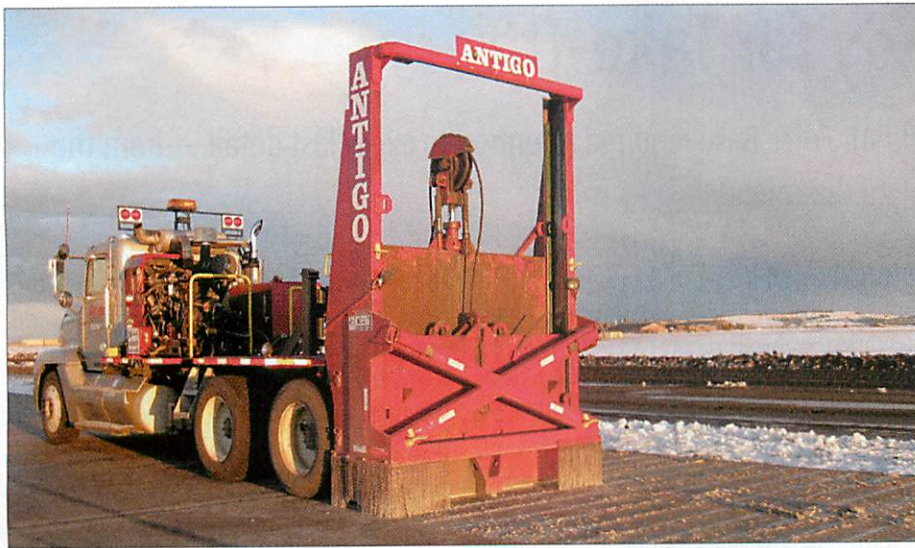
Construction of the new runway at Fairchild Air Force Base was completed on schedule in November 2011.
