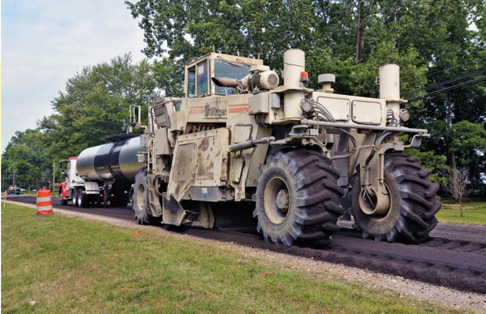
Left (top to bottom): (top) A Wirtgen in-place recycler mixed the RAP on-site; (middle) Padfoot roller compaction in action; (bottom) Virgin asphalt was laid on top at 3.5 in.
