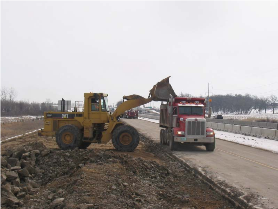
Front end loader loading broken concrete in dump truck for transport to crushing site.
