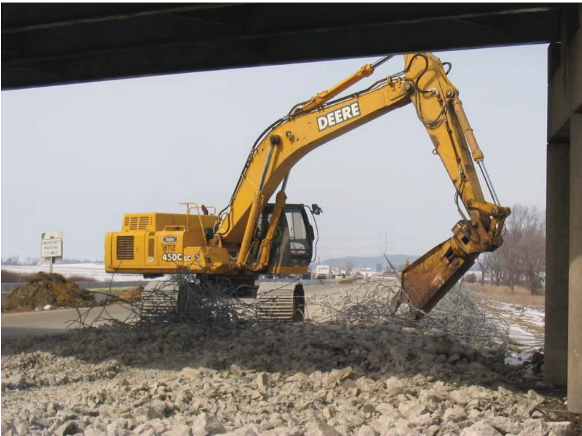
Excavator with shears attachment cutting reinforcing bar to manageable size for hauling to recycling center.
