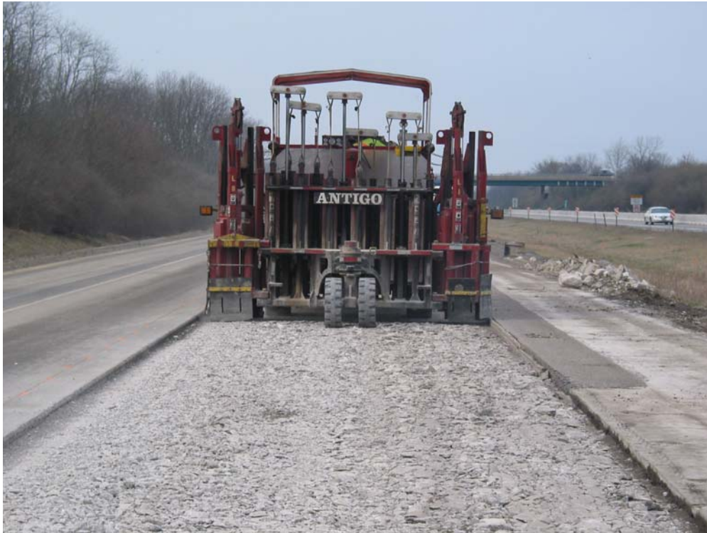
MHB Badger Breaker® rubblizing continuously reinforced concrete pavement (CRCP) on I-70, Clark County, IL during 2003. 37 lane miles of rubblization and HMA overlay.
