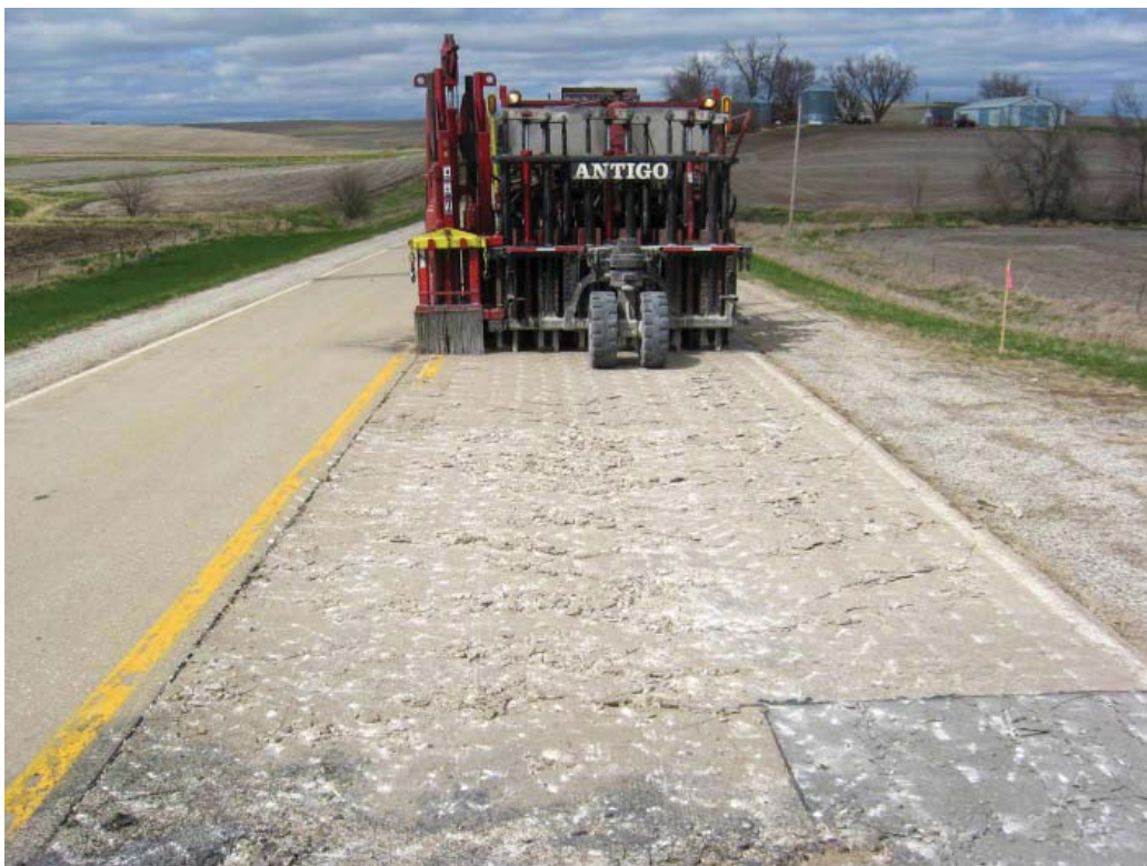
Modified Rubblization—significant spalling
