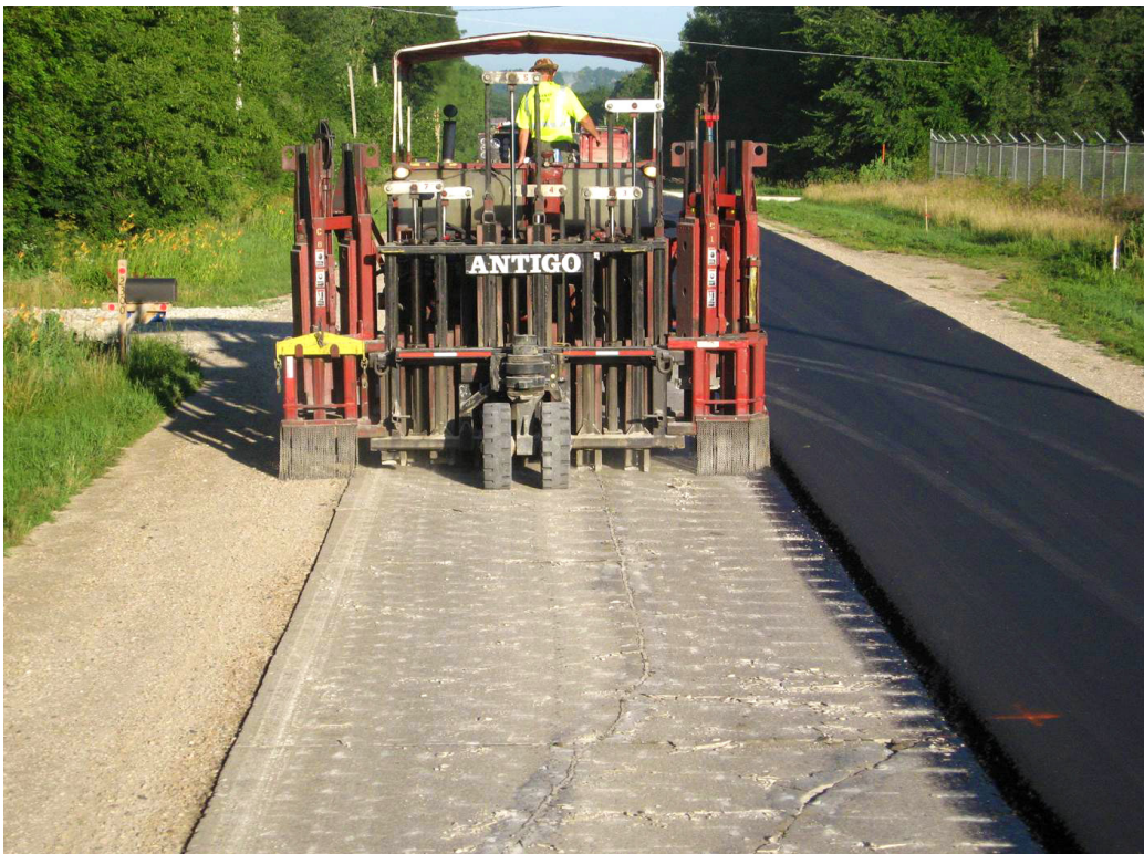
Modified Rubblization – occasional spalling
