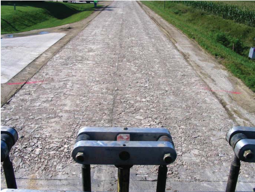
Modified Rubblization—significant spalling
