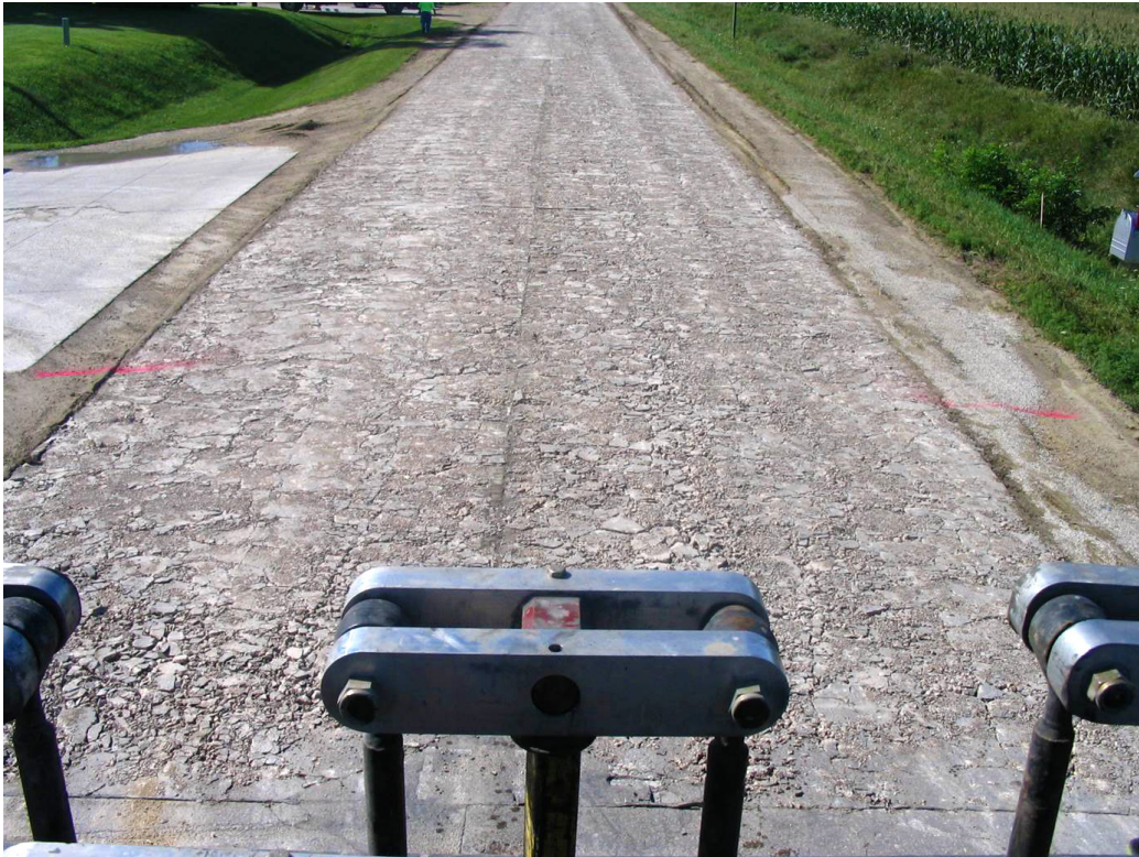
Modified Rubblization – significant spalling
