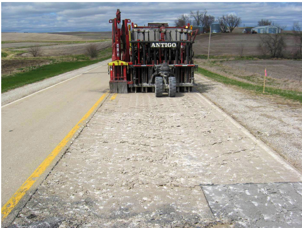
Modified Rubblization – significant spalling
