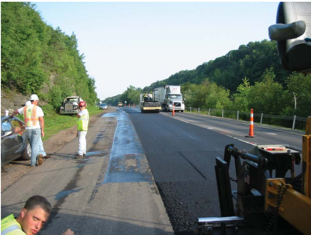
Finishing paving early next morning. Note that first lift of new asphalt overlay matches up with existing overlay on adjacent lane.
