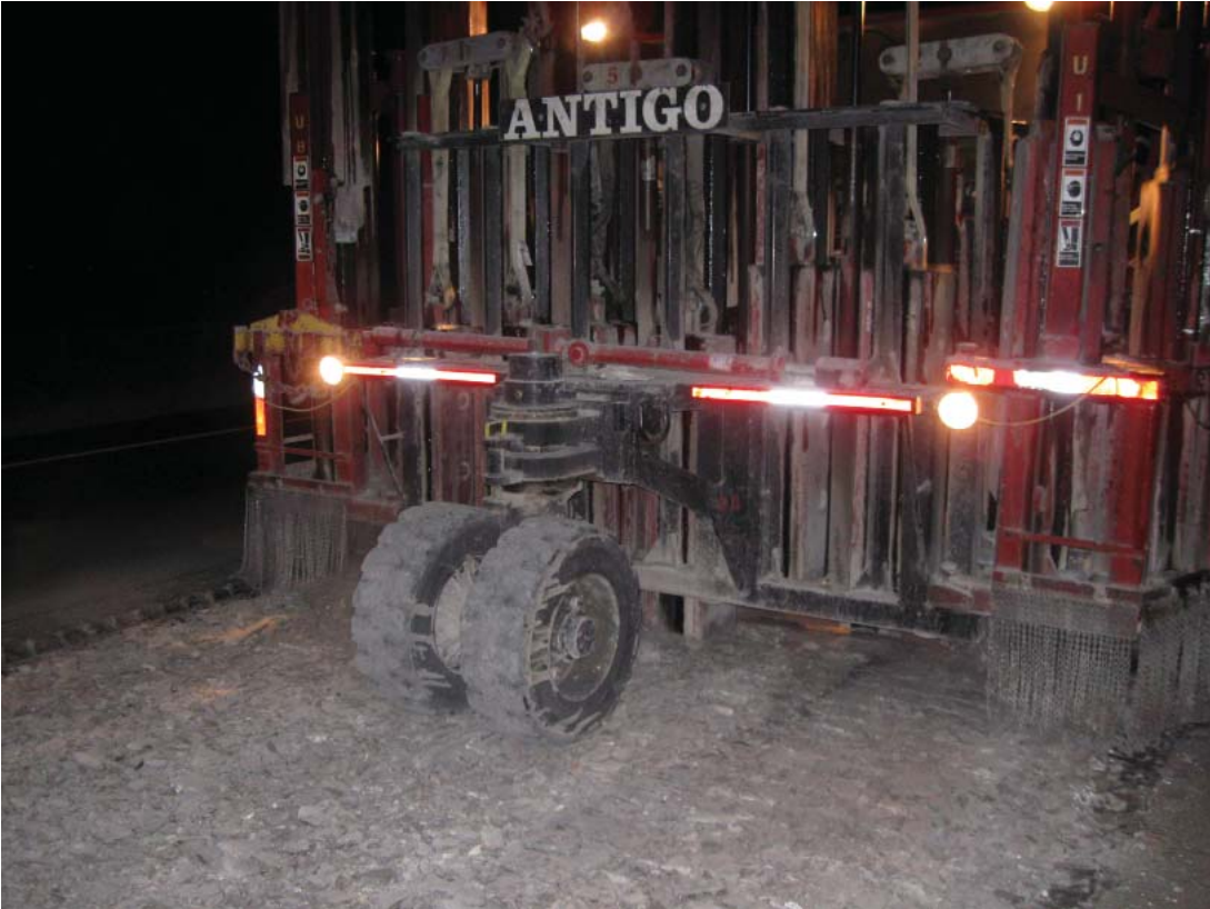
MHB rubblizing second lane. Note first lift of asphalt overlay on previously rubblized lane to the left.
