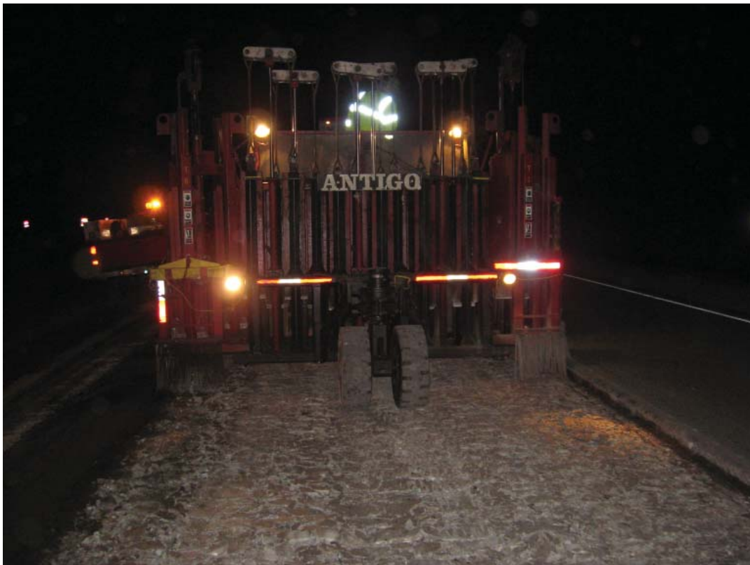
MHB Badger Breaker® rubblizing at night after existing asphalt overlay milled off. Note existing asphalt overlay in place on right lane.
