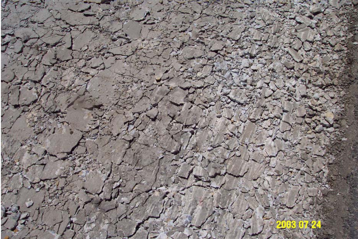
FIGURE 5 Note the “flaky” rubblized PCC surface.
