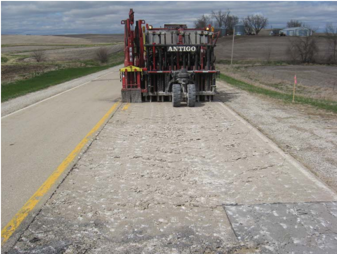
Typical modified rubblization - significant spalling.
