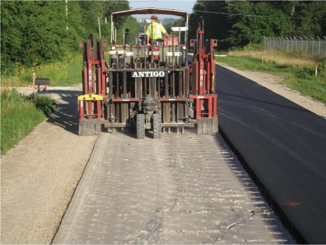
Typical modified rubblization - occasional spalling.
