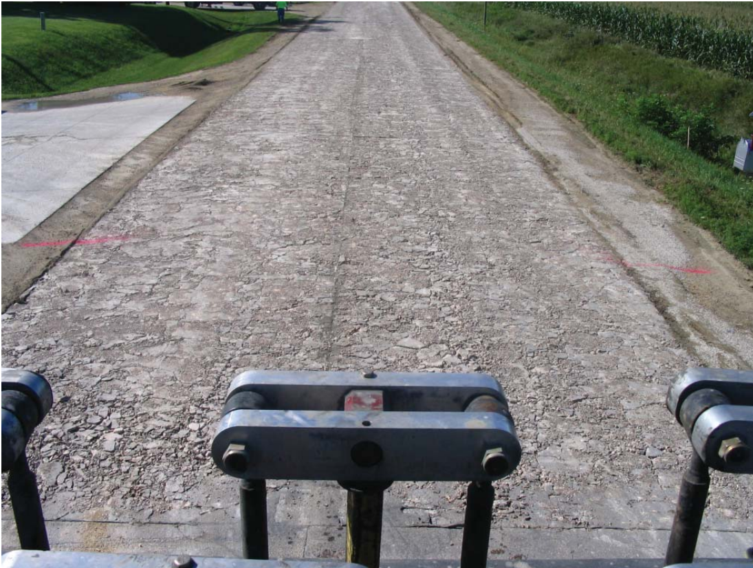
Example of more significant spalling.
