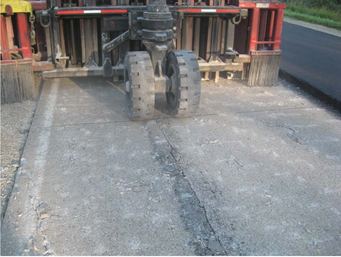
Clearly visible cracks.
