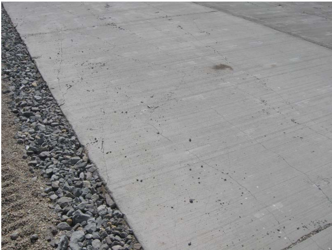
Visible hairline cracks.
